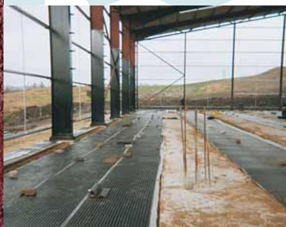
Ventilation System - Waste Transfer Station
